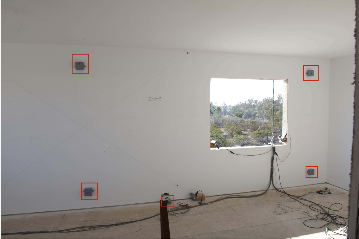
Figure 4: Sensor location on the West side wall: Interior wall of the 2nd floor. The squares indicate the locations of the sensors
